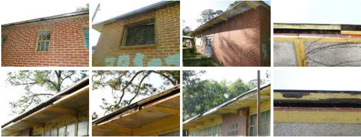
7). Most of the windows on both buildings are damaged. The frames are delaminated from corrosion. The glass is missing and shattered in most windows.
