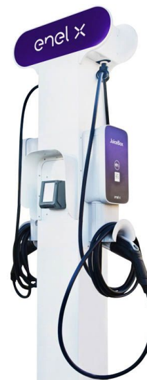
Enel X JuicePedestal Level 2 Charger
