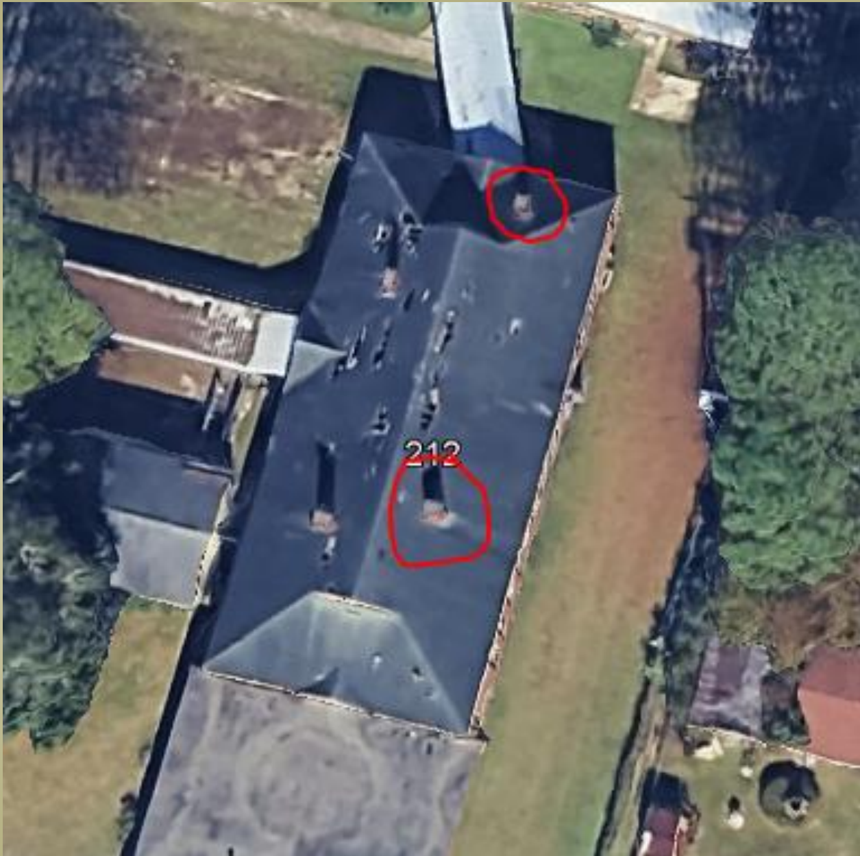
Removed Damaged Stacks on Back of Building
